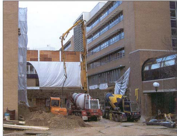
Concrete trucks pump the large amount of concrete needed for various components within the cyclotron facility.
