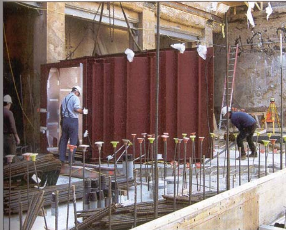
The construction team works to install the massive vault door. The door was filled with concrete, as well.
